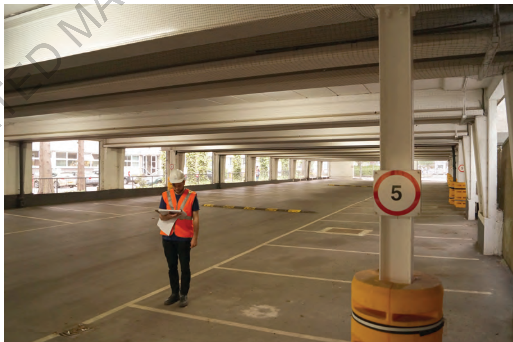
Figure 10.1 Routine inspection using a prepared checklist, while the car park is not in use. Checking the presence and condition of impact protection jackets that have been retro-fitted to structural steel columns (courtesy of Mott MacDonald Ltd)
